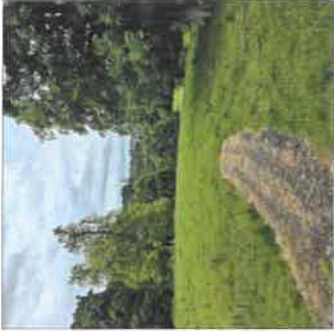
PHOTO P2: CABLE ROUTE FROM POC
