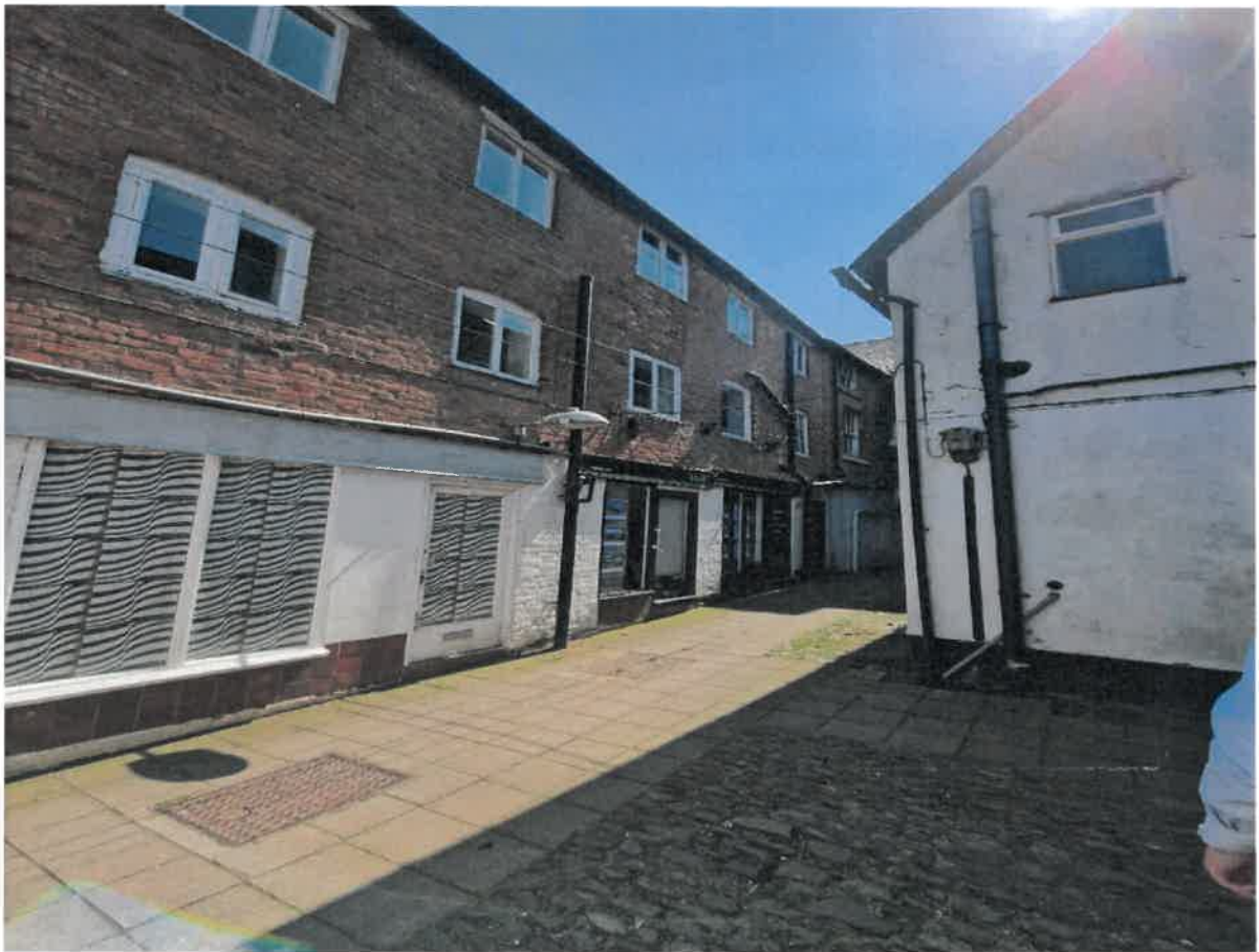
Casement timber windows to Hopkins Passage to be replaced as part of the works.
